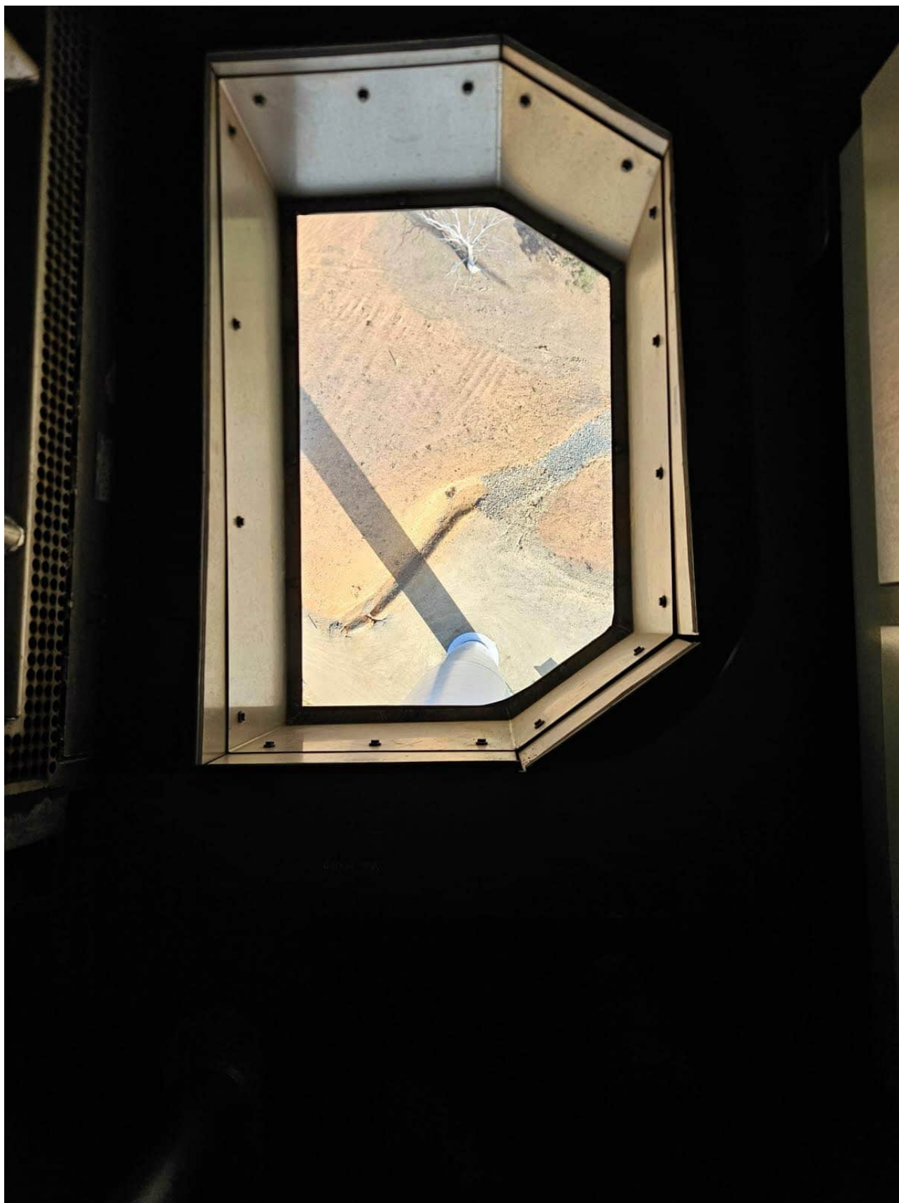
Figure 12: Hatch that Nankeen Kestrels were entering through the base of the nacelle at WTG 01. Image shows inspected hatch area where no nests or birds were present prior to making the turbine operational again.
