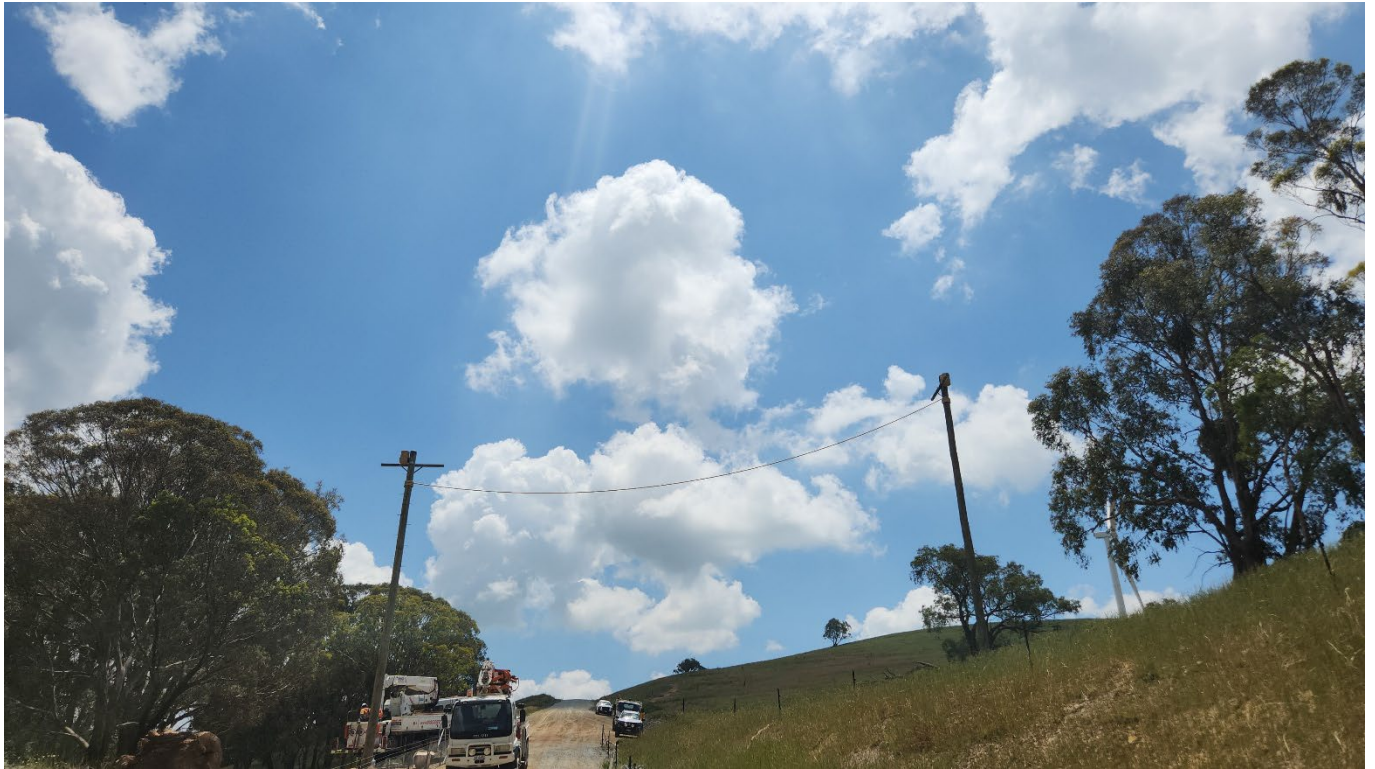
Figure 5: Glider crossing inclusive of poles, rope bridge and Habitat boxes installed at Flyers Creek Wind Farm
