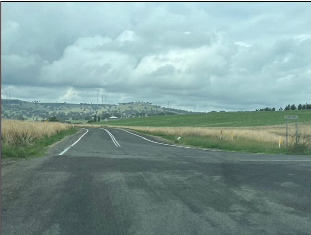
Plate 10: View of road upgrade and rehabilitation works at the intersection of Panuara Road and Errowanbang Road. All works completed were conducted in consultation with Blayney Shire Council with good results evident.
