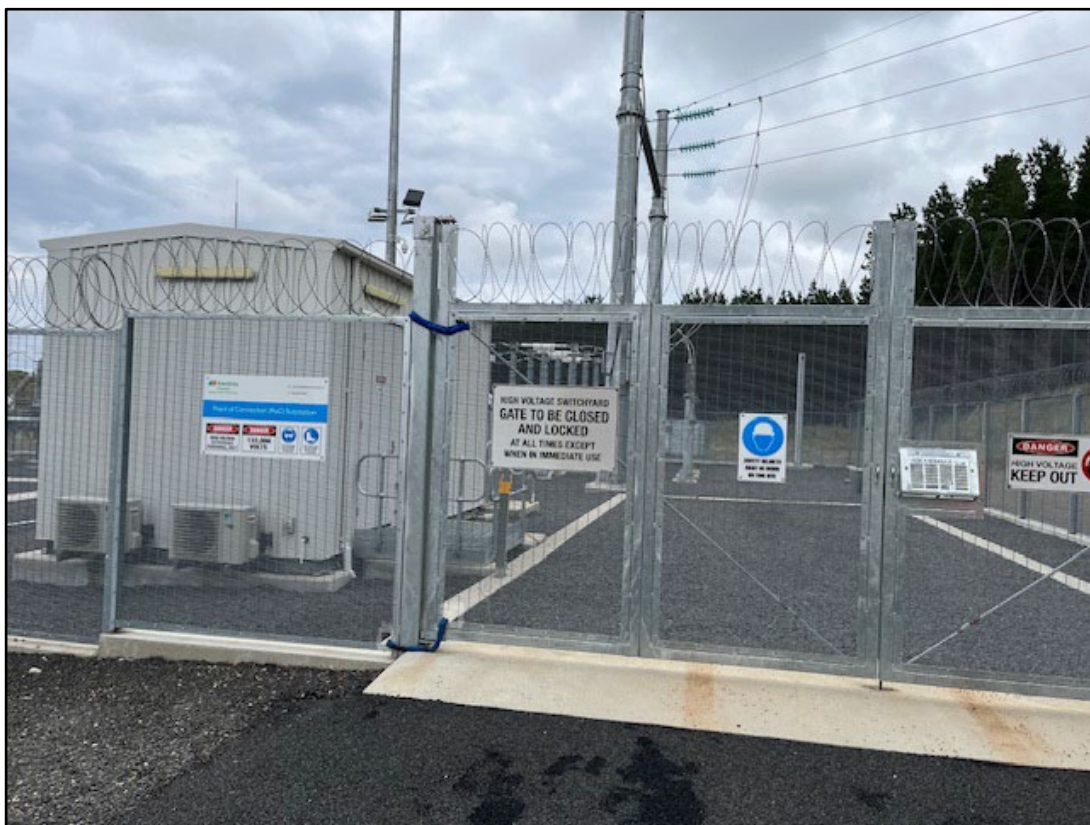
Plate 6: View of site infrastructure (point of connection). Building colours were noted to be of low-reflectivity and off-white colour. Lighting was confirmed as low-intensity and only used on an as-needed basis. In particular, it was not dusk- or movement-activated to ensure that no lights were operating at night. Well established Asset Protection Zones were noted to present at all viewed infrastructure locations.
