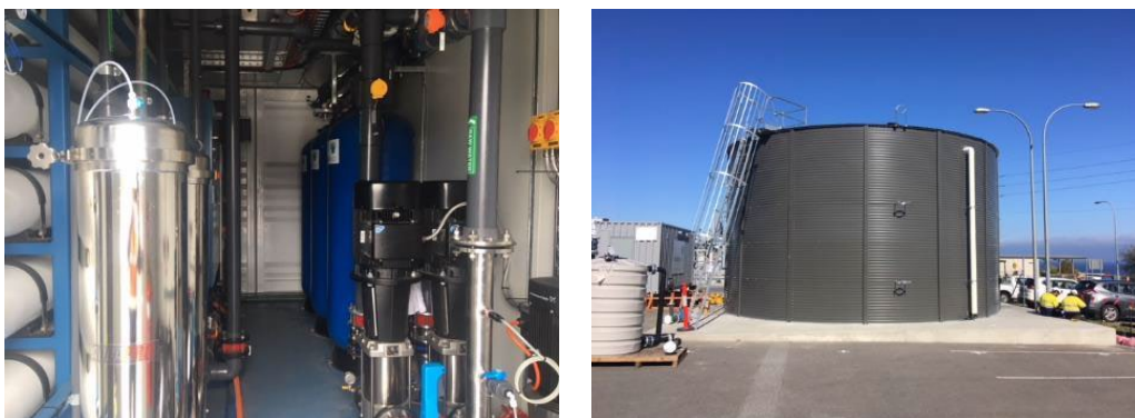
Figure 11: RO Water Treatment Plant and Raw Water Storage Tank
