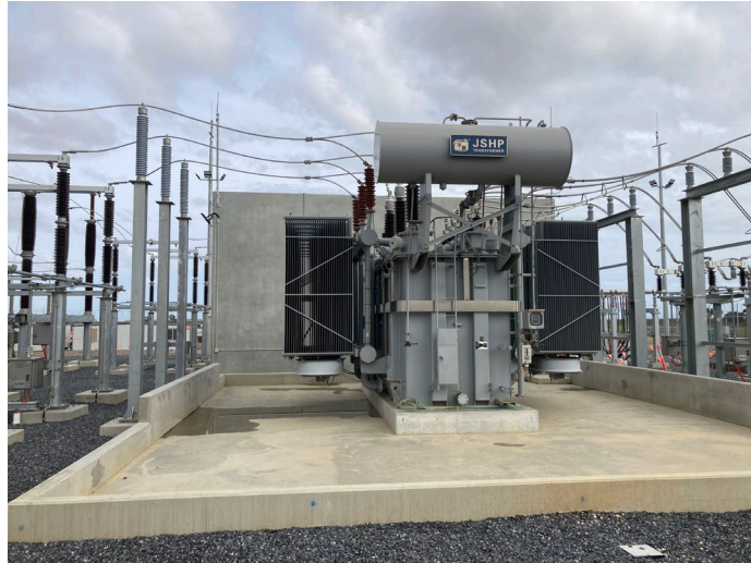
Figure 10: Main transformer at BPS
